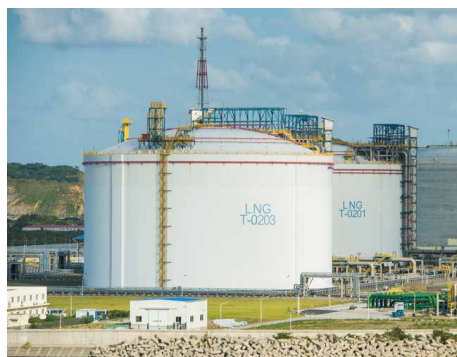
Liquid level tank
